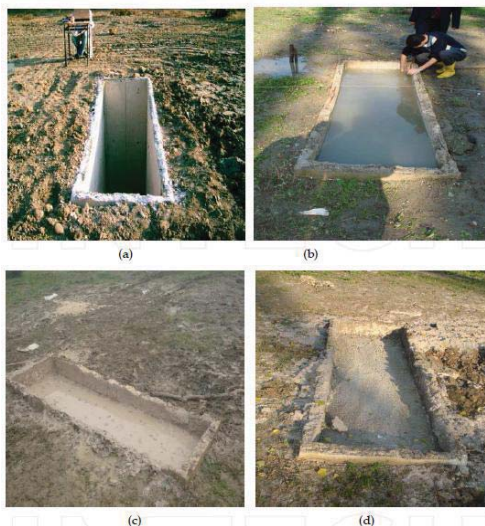
Figure 6. Trench-type insulating barriers: a) open trench, b) pre-filled trench with water, c) trench filled with bentonite, d) concrete ditch
