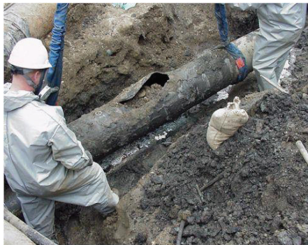
Figure 2. View of a broken crude oil pipeline
