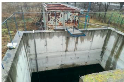
Figure 1. The Treatment plant Daia Romana 1
