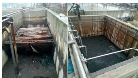
Figure 2. The Treatment plant Daia Romana 2
