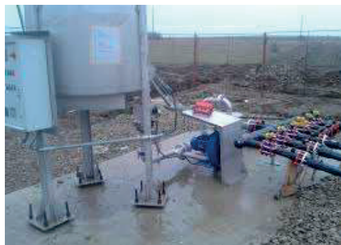
Figure 3. The biogas installation from Sibiu County
