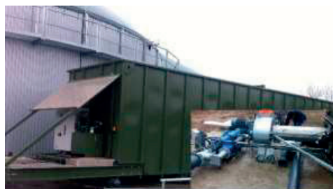
Figure 9. Grinding system installed at the exit of solids feeding system
