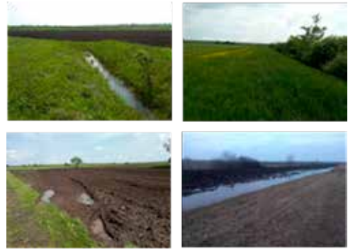
Figure 9. Clogging of ducts and prolongation of excess moisture
