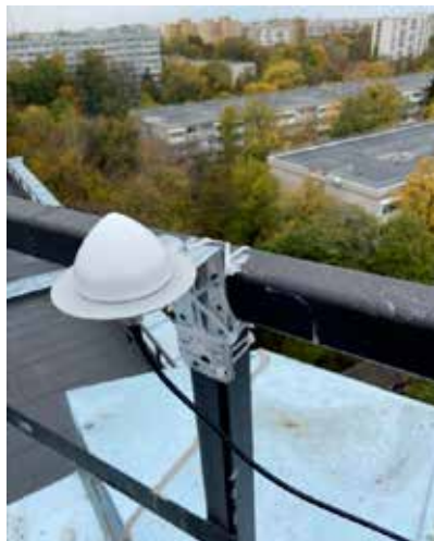
Figure 2. Photo of a GNSS antenna on a roof
