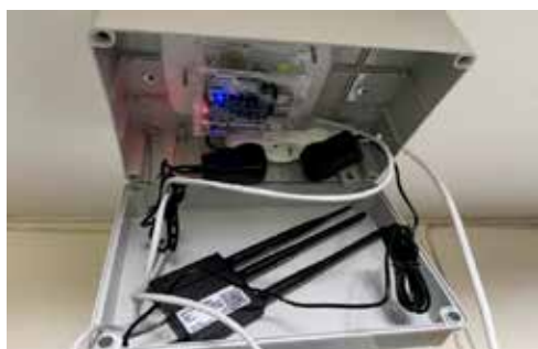
Figure 1. Photo of an installed RS4D sensor setup
