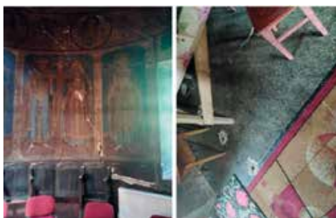
Figure 3. Deformation and Cracks in the Different Structure inside the Church Adormirea Maicii Domnului, Perișoru
