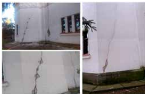
Figure 2. Deformations and cracks on the Brick Walls of Church Adormirea Maicii Domnului, Perișoru
