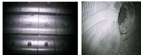
Figure 3. Cascade shields (detail) and slots in the partition wall with ventilation ring (detail) - chamber I
