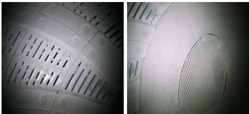
Figure 6. The slots in the mill outlet wall (detail) and mill outlet grate (detail) - chamber II
