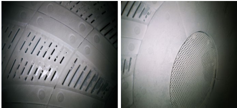
Figure 6. The slots in the mill outlet wall (detail) and mill outlet grate (detail) - chamber II
