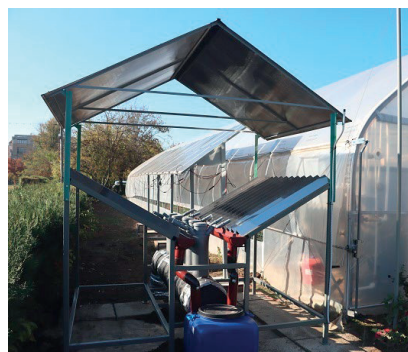
the outdoor unit (the collector)
