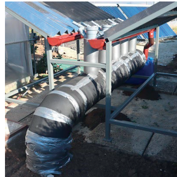
warm air piping
