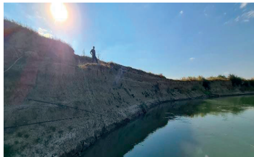
Figure 4. Riverbank erosion in the study area (original)
