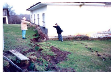
Figure 8. Ground failure near the building school, Duzce -1999 (INCERC photo)
